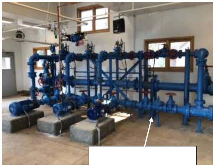
Figure 7-6 – Base 1 BPS Photo
